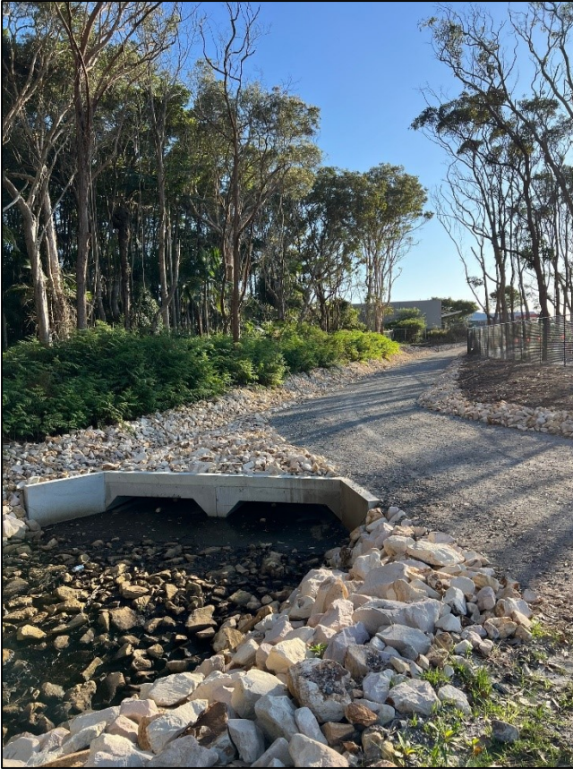
Photo 4: Existing approved stormwater infrastructure in C2 zone (see Figure 4)
